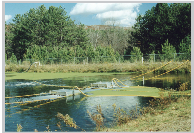
Two unit system installed at Quaker Lake WWTP.
