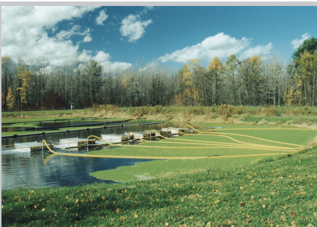
Six unit system installed at Laurel Lake WWTP.
