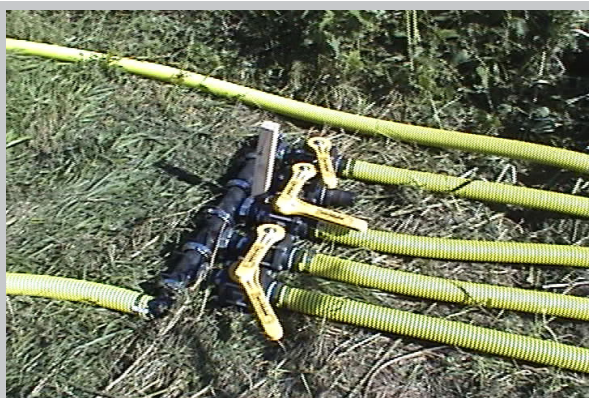
On shore manifold constructed of ultra strength polypropylene valves & fittings (photo taken during start-up).
