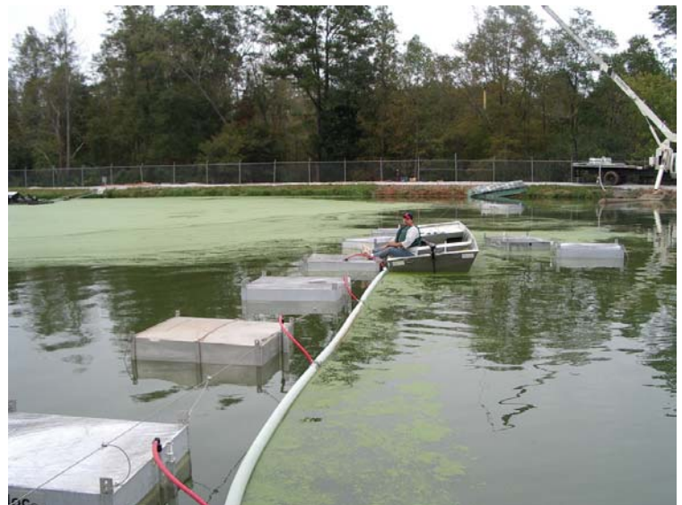
Bio 2 Bloc units FLOAT into place. System is moored between cables from shore to shore.
