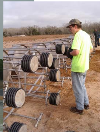
Ballast weights installed at bottom of each diffuser leg, for operational stability on the "double-puss"
